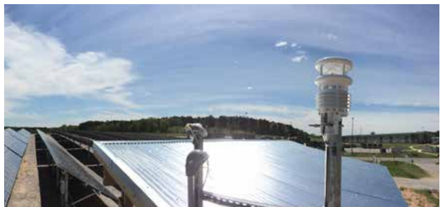
LUFFT WS500 monitoring the solar power plant in Fort Pickett. Image: Virginia National Guard
